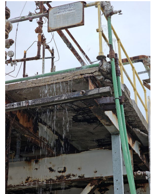
Flushing Flow Lines
