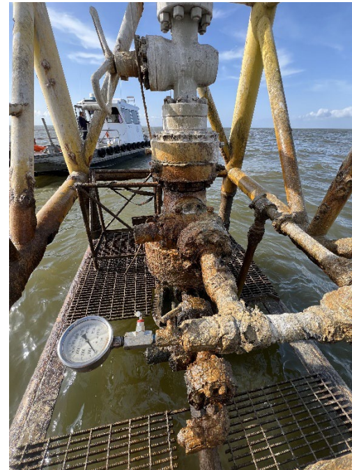
Needle Valve & New Gauge Installed
