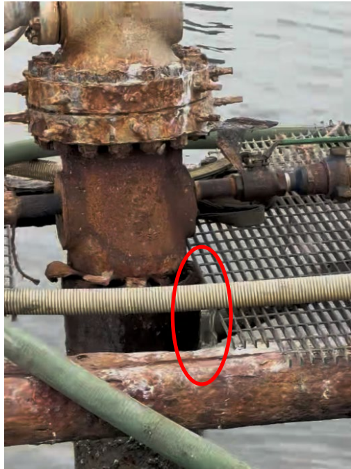
Leaking Drive Pipe
