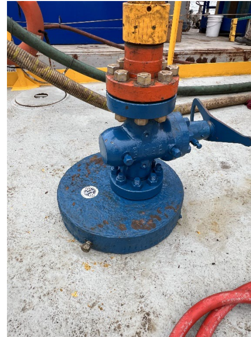
Obsolete Wellhead Design (limited replacement options if non- functional)
