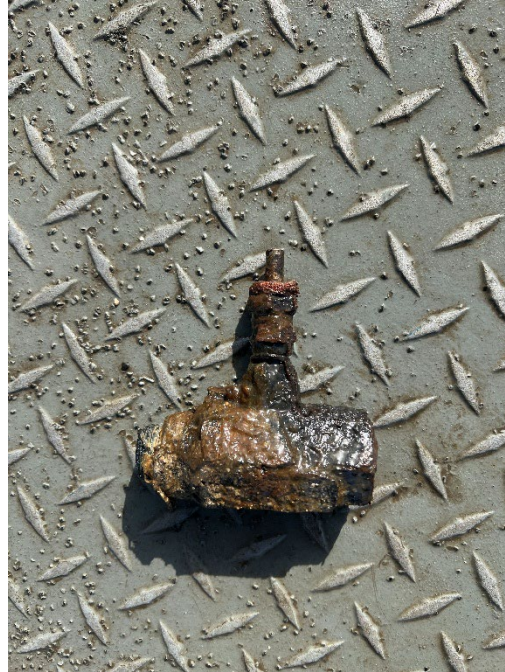
Corroded Needle Valve
