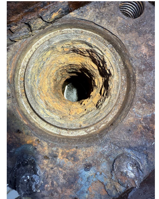
Internal Scale Buildup
