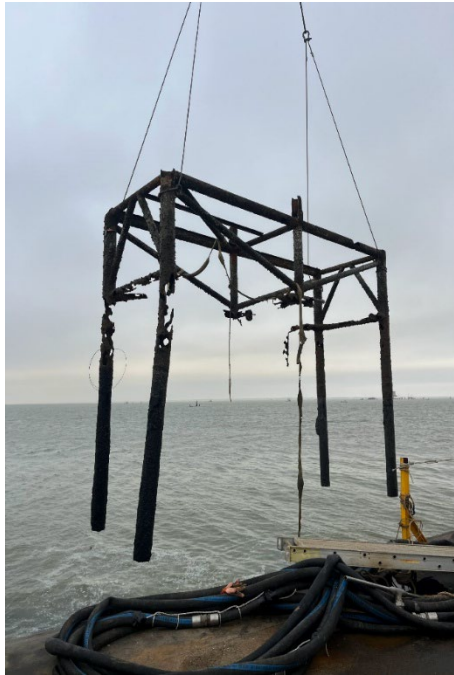
Degraded Platform Structures
