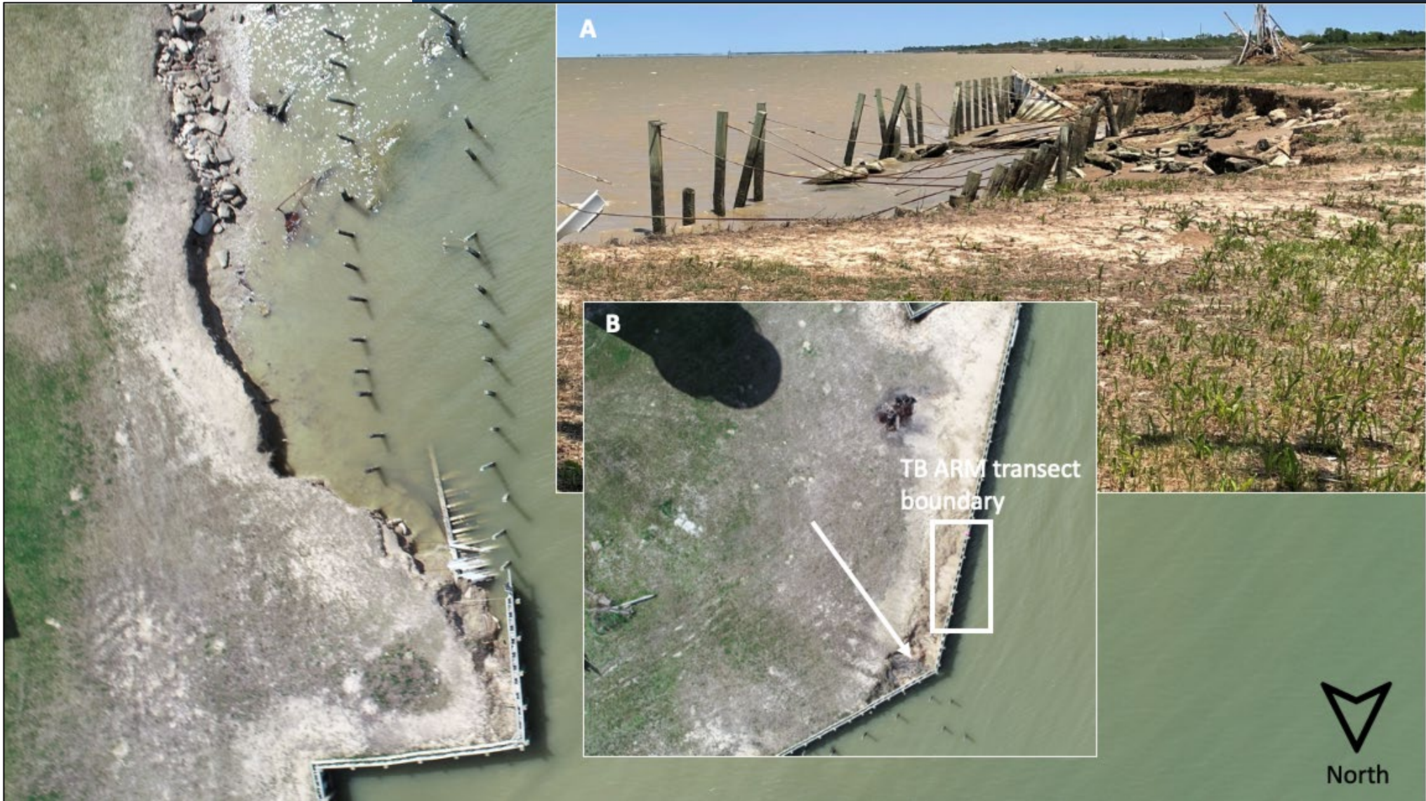
Failing sheet pile bulkhead at Trinity Bay. Inset A shows the damage from the ground, looking toward the south. The study boundary for TB ARM is immediately south of the damaged area (Inset B), on the same bulkhead, where undermining is also becoming evident.
