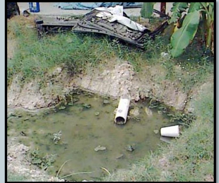
FAILING ON -SITE SEWAGE SYSTEMS
