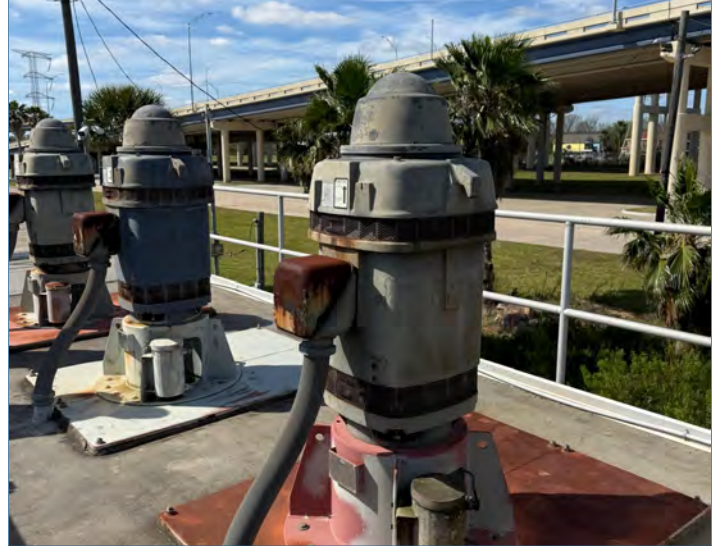
Photo 13. Existing primary pump equipment on the elevated pump station platform.
