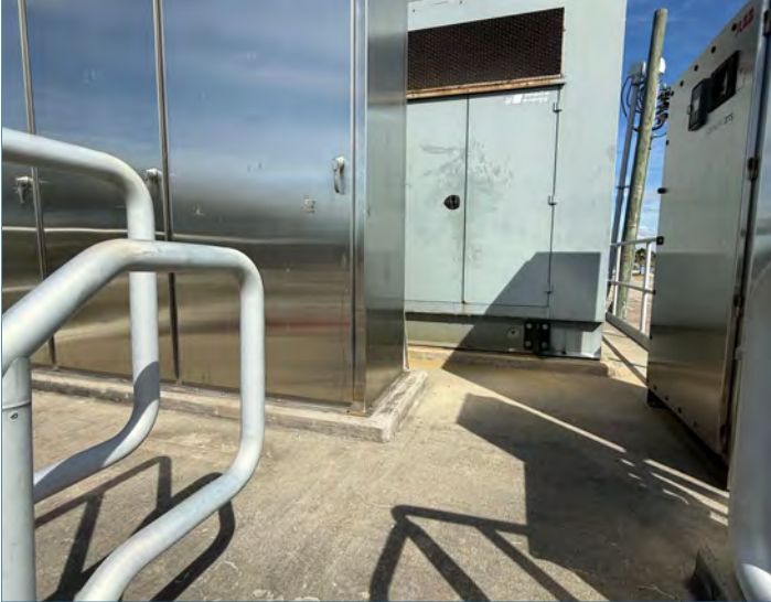
Photo 16. Existing generator and electrical/mechanical equipment serving the pump station.
