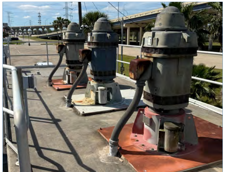
Photo 15. Wide view of the three primary pump units and elevated operating platform.
