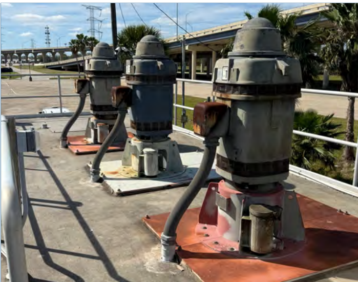
Photo 14. Existing pump equipment and maintenance platform area.
