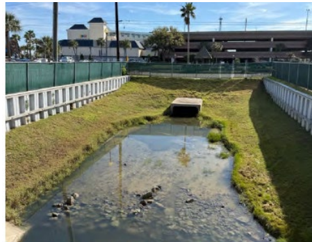
Photo 8. Existing forebay/inlet area with ponded water and visible sediment accumulation upstream of the pump station.
