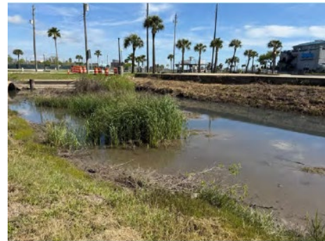
Photo 25. Receiving channel near the downstream end with emergent vegetation and accumulated sediment.
